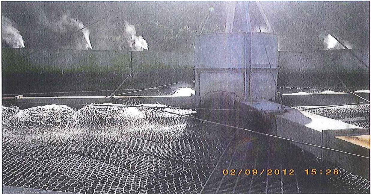
Biotower #1 Distribution Arm Condition Assessment. Odor control equipment operating on the tower wall in the background.
