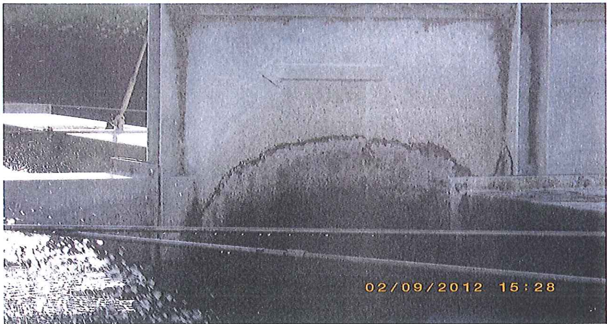
Biotower #1 Center Column Condition Assessment. Algal growth forms on the center column from the distribution of aerated primary effluent.
