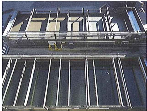
Existing DAF's (top view)
