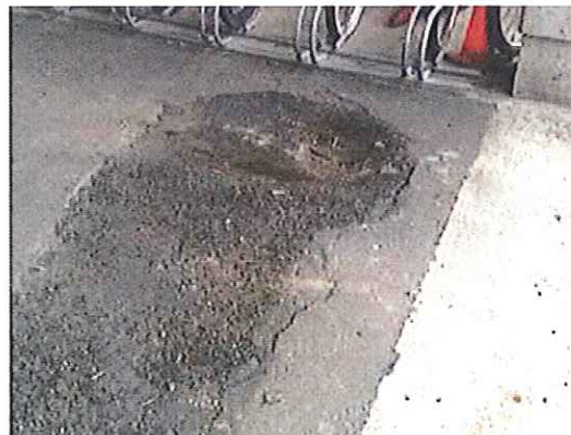
Failed one-year old repair to asphalt slab.
