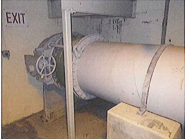
Primary Effluent Pipe emerging into gallery
