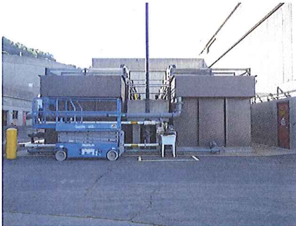
Existing DAF's (end view)
