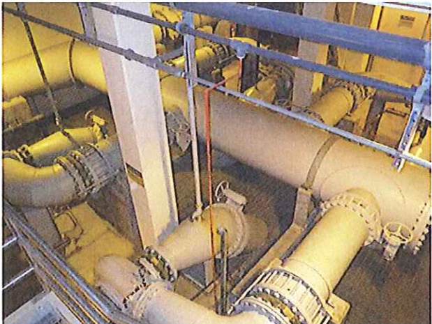
RAS pipe manifold
