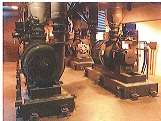
Existing Original Centrifugal Blowers
