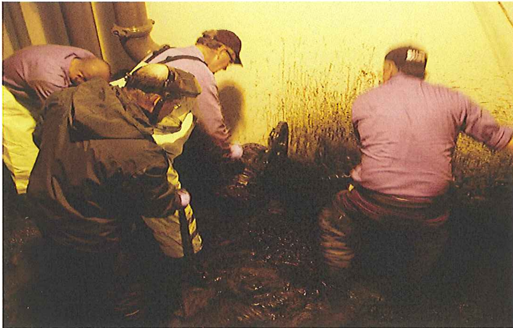
Staff unplugging a line into Digester #1
