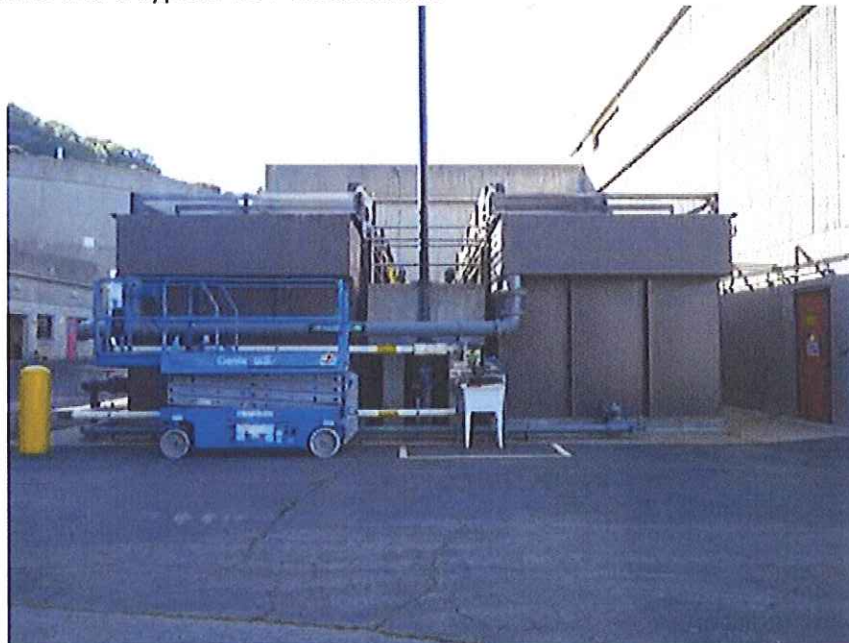
Existing Dissolved Air Flotation Tanks
