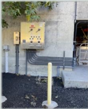
Original Control Cabinet
