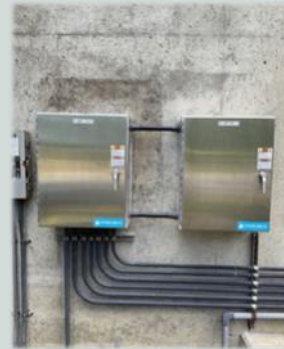
New Control Cabinets
