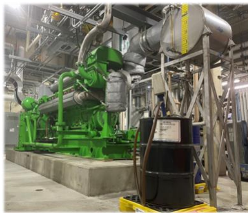
New cogeneration engine in operation.
