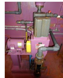
Originally Installed Ferric Chloride Pump
