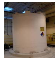
Sodium Hypochlorite Tank #4
