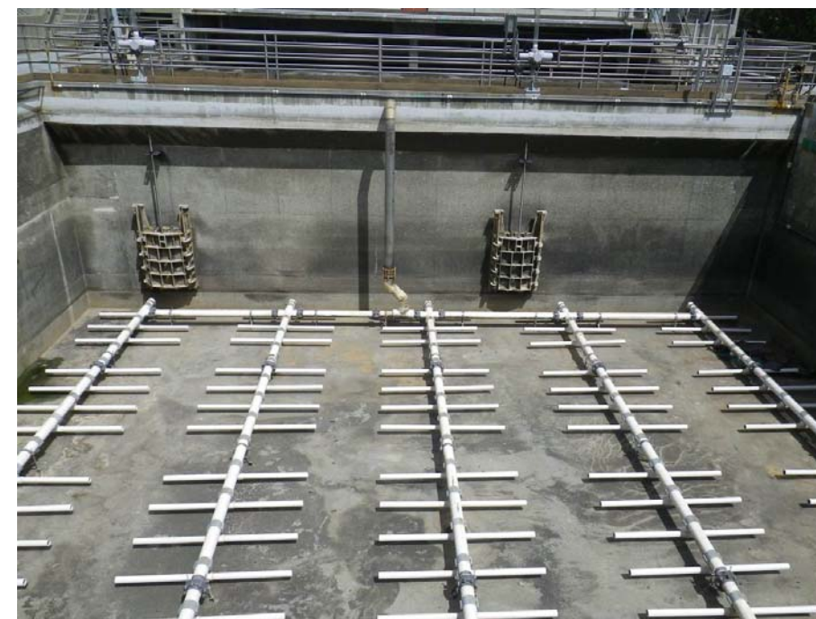
Aeration Basin #1 Diffusers
