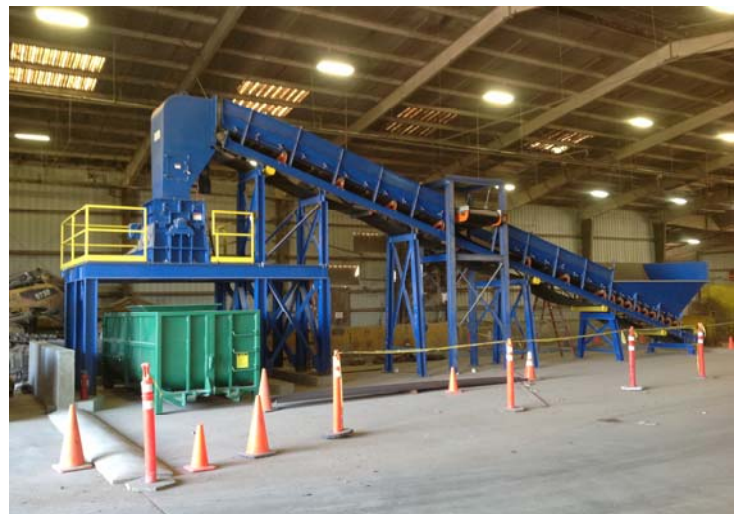
Marin Sanitary Service Food-to-Energy Equipment.
