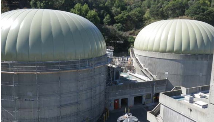
Digesters No. 1 and 2 with membrane covers in operation.
