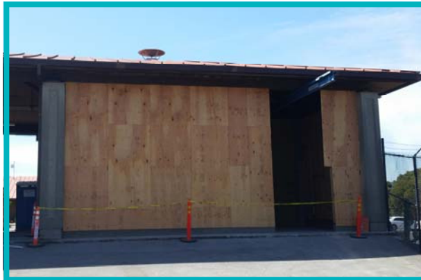
Above and to left: Open side of the Maintenance Building being enclosed for storage (before and during construction).
